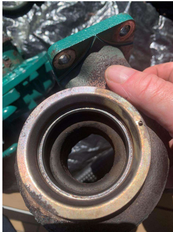
Turbo Exhaust inside Chamber before the Turbine 2. No Soot Accumulation but Corrosion Where the Turbine let the Hot Gaz into the Elbow. Please note also the alignment pin.
